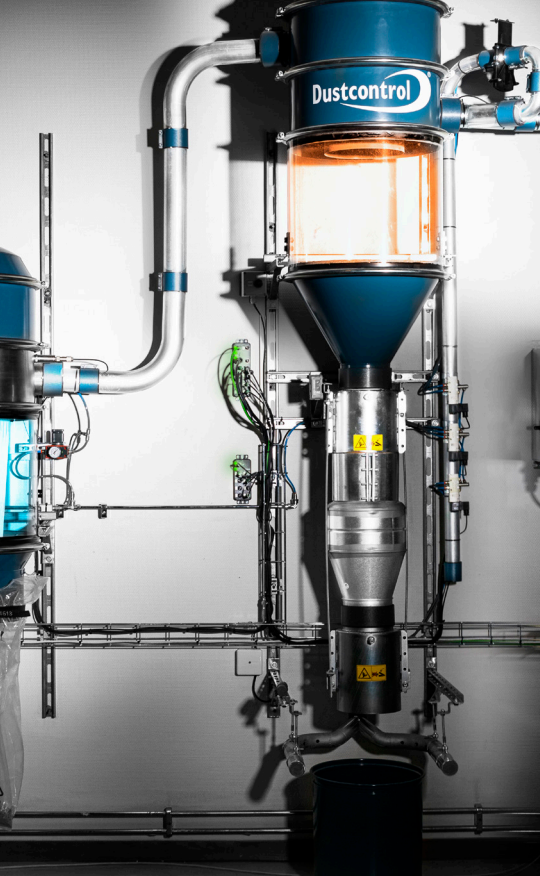
In Norsborg, we have a test facility indoors where you can see how our comprehensive solutions clean the air.
